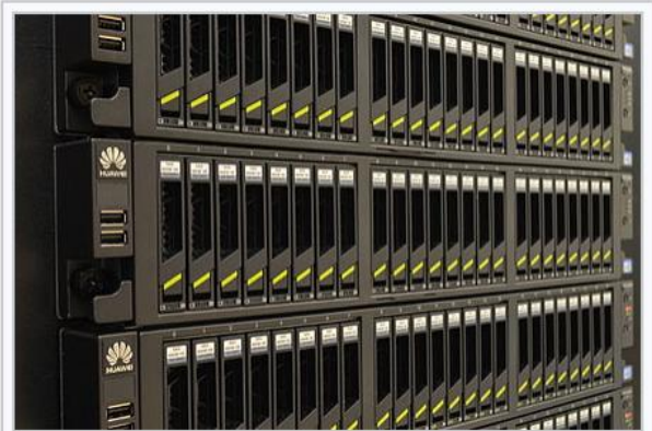
Storage servers with 24 hard disk drives and built-in hardware RAID controllers supporting various RAID levels
